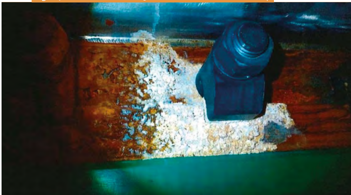
Figure 71 · Corrosion at Mochovce-3 Reactor Pressure Vessel Prior to Startup
